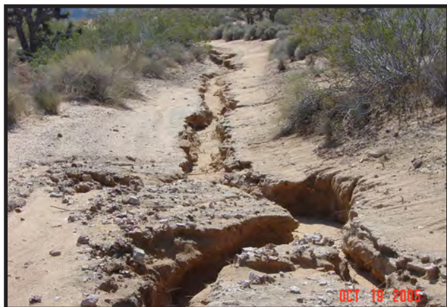
Figure 4. Severe erosion on Steep Trail at KER-376.
