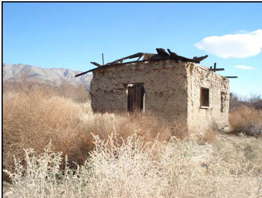
Fig. 7. Bailey Earthen Structure (Bailey Cabin; P-37-02812) before the protective roof was placed over it. View to NE. Photo by J. Schneider.
