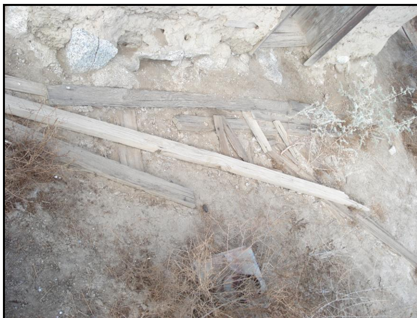
Fig. 8. Typical view of materials fallen around the base and foundation of the Bailey Cabin before mapping and collection. Metal stovepipe part lies covered by brush and debris. Door opening at top right. View of the eastern aspect of the cabin, to NW and down. Photo by J. Schneider.
